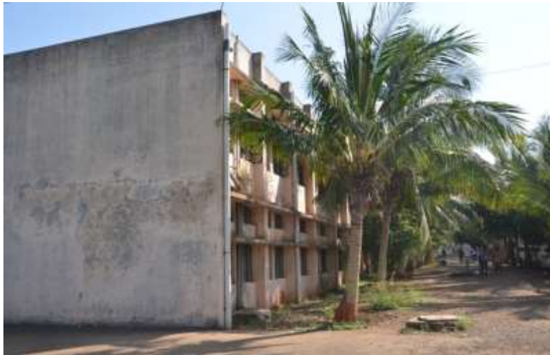
Roof top Rain Water Harvesting (Back Side of Library Building)
