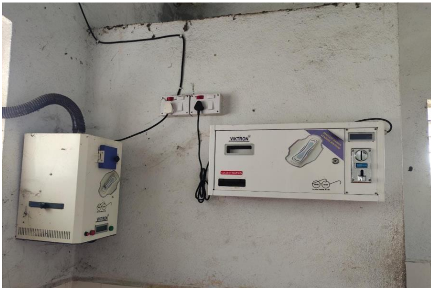
Sanitary Pad Vending Machine And incinerator
