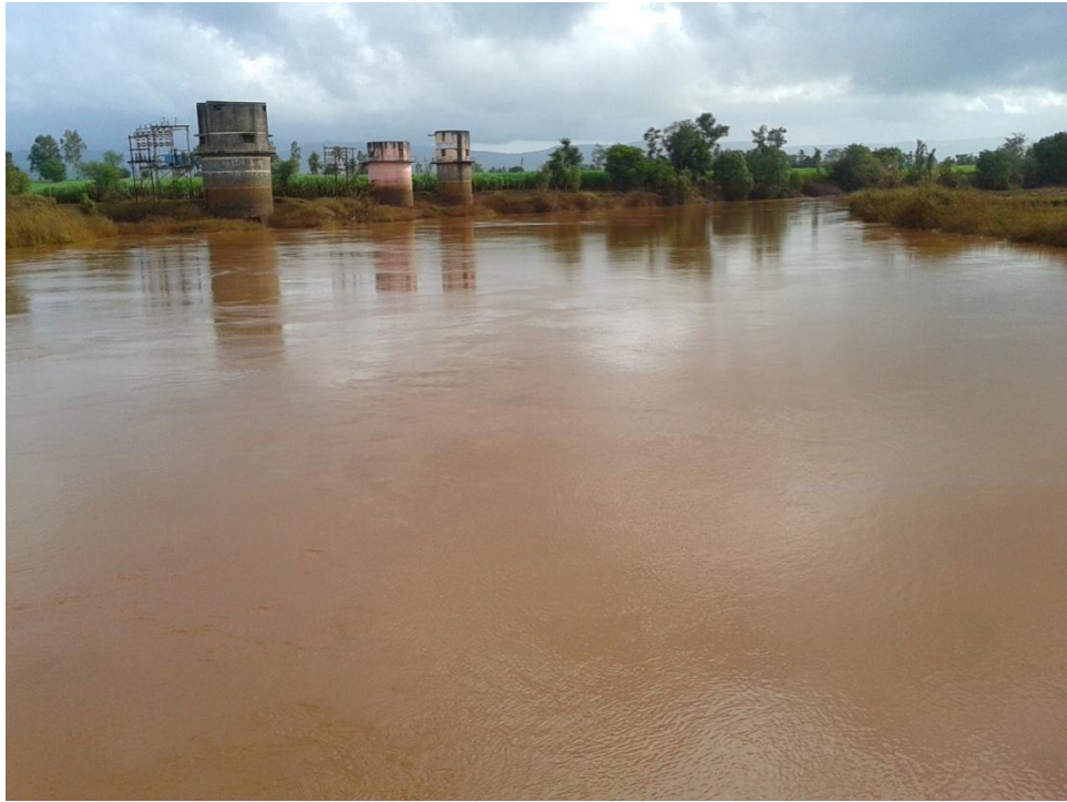
Photo Plate. 3. Flood situation at Kakhe Site.
