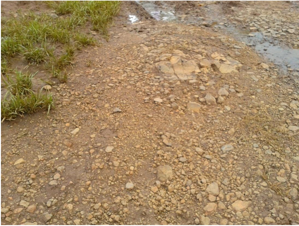
Photo Plate 7. Erosion of soil due to flood.
